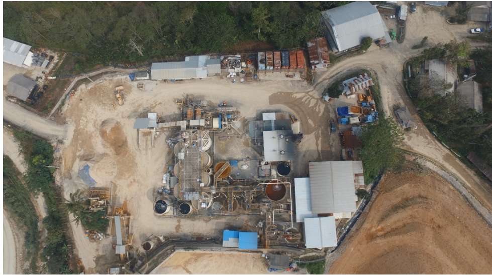
▼ Way Linggo Processing Plant
